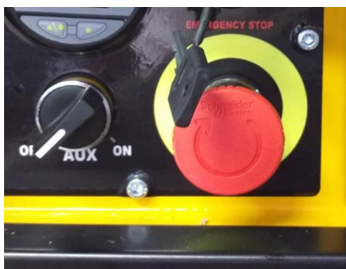
9. Ground control panel emergency button
