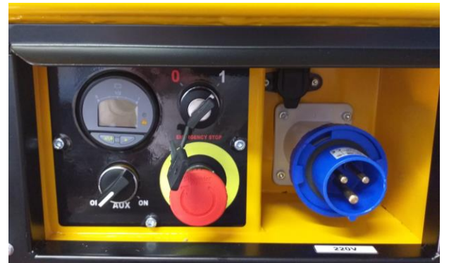
6. Ground control panel
