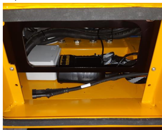
12. Remote control battery recharge compartment
