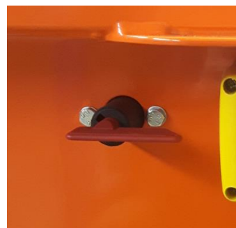
14. Battery disconnect switch
